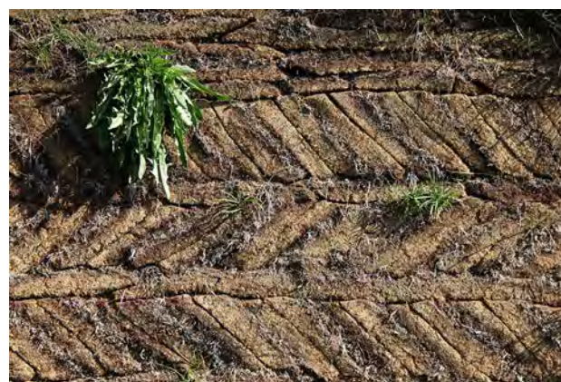
Fig. 3.8: Different building techniques were used according to the quality, accessibility, and functionally of the turf. Here small pieces of turf were used.
